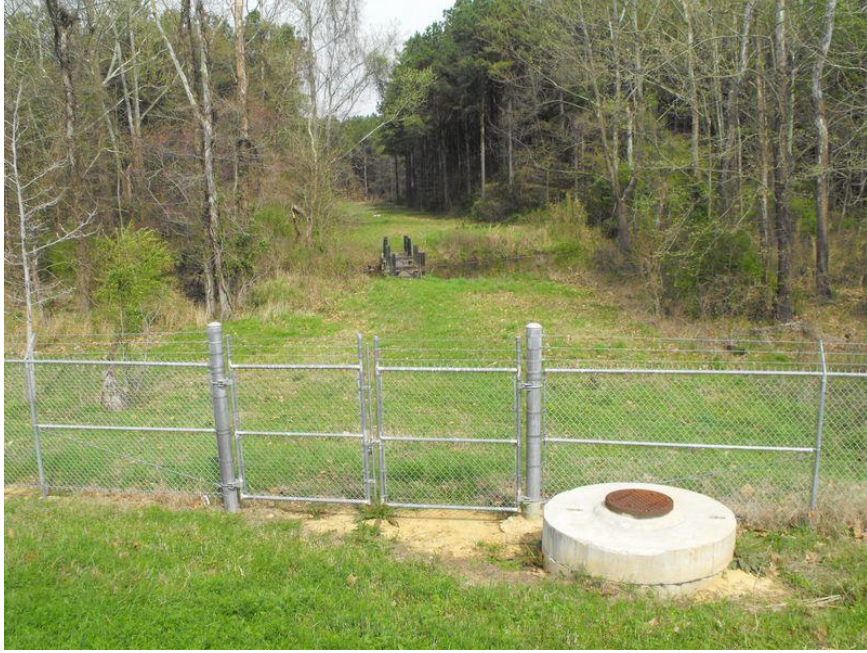
City of Crossett Manhole and Wastewater Pipe Crossing Coffee Creek
