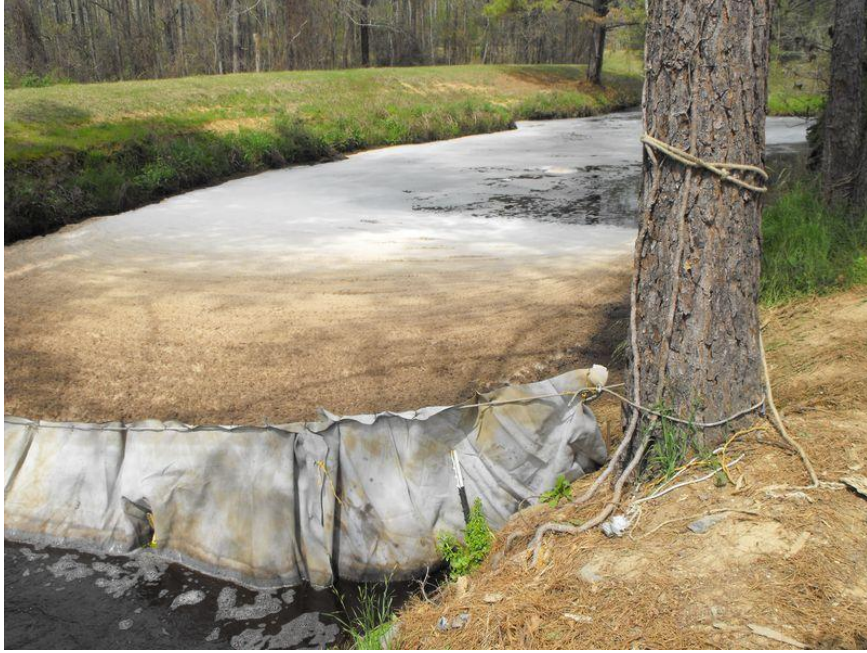
Foam Curtain Control in Aeration Basin Channel Prior to Outfall 001
