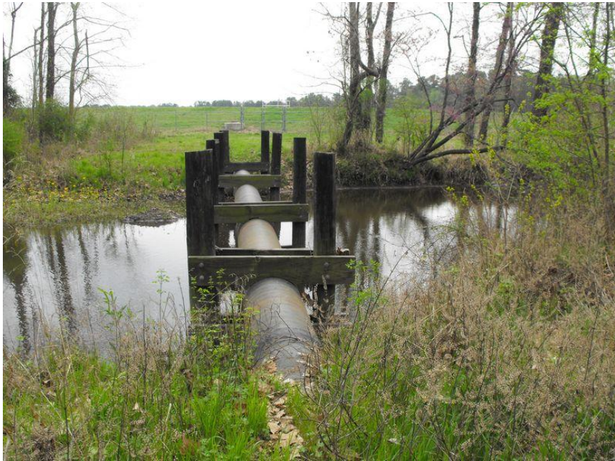
Close Up View of City of Crossett's Wastewater Pipe Crossing Coffee Creek
