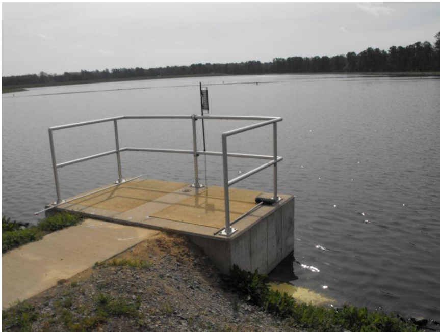
Close Up View of City of Crossett Wastewater Treatment Pond Outfall Structure
