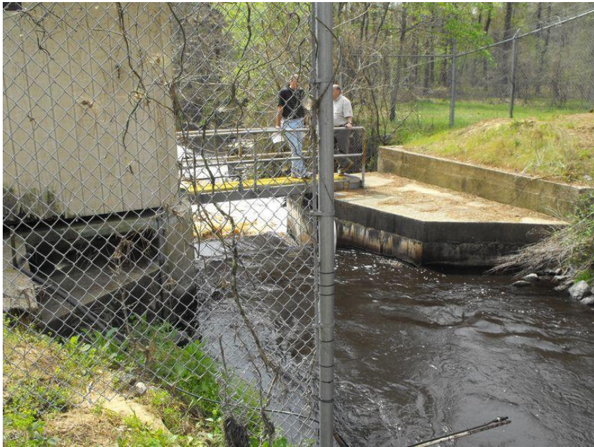
Looking Downstream of Curtain and Defoamer Pipe at Outfall 001 – No Foam to Flume
